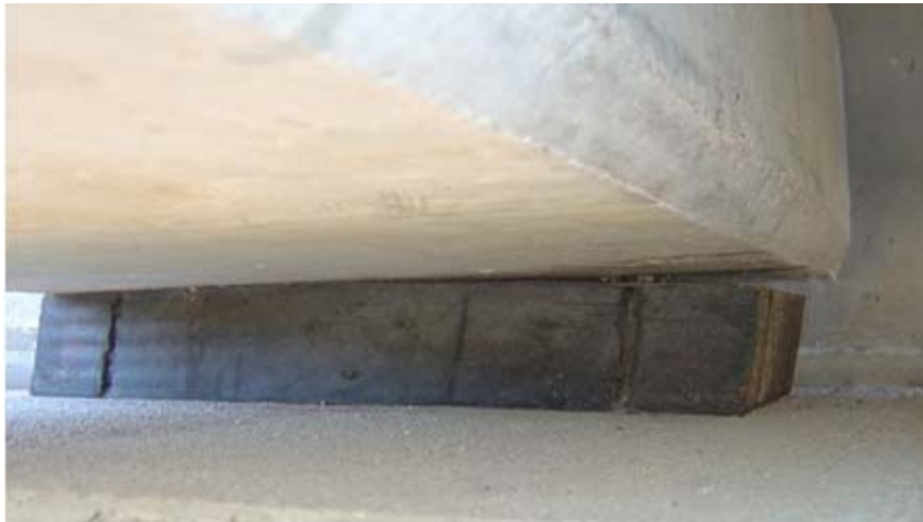
Figure 6.2 Lift-off of Fascia Beam at Hutto Concrete Bridge
