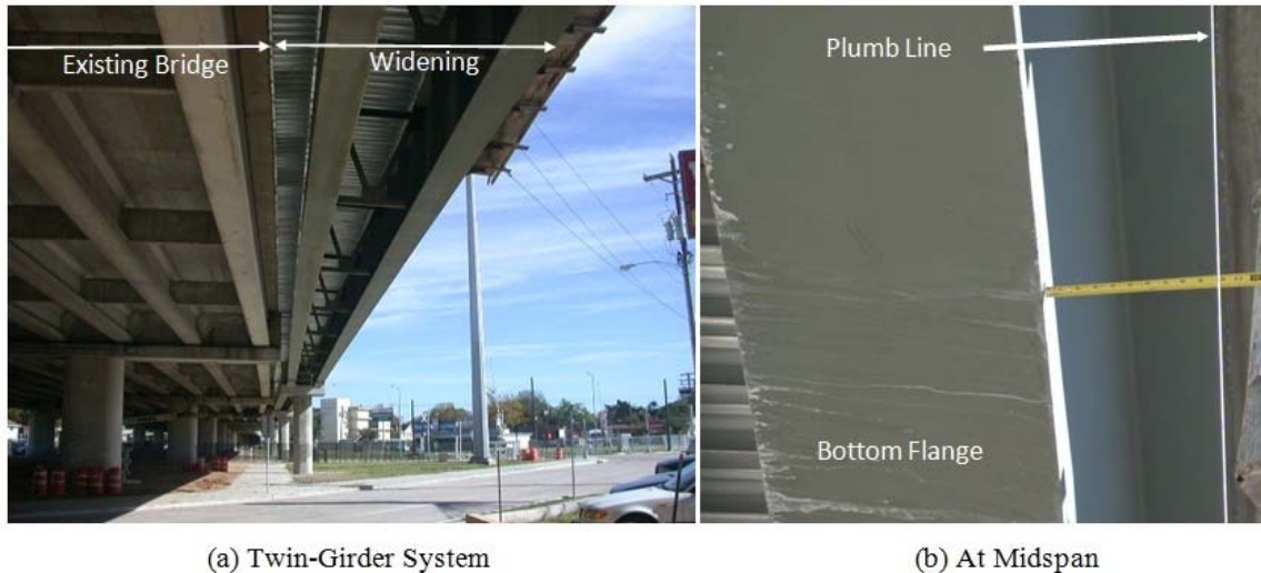
Figure 2.13 Twin-Girder Widening with Excessive Girder Rotation
