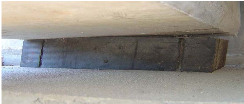
Figure 2.15 Lift-off of Fascia Girder from Bearing Pad
