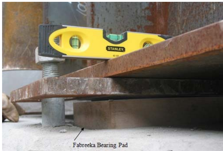
Figure 4.19 Fabreeka Bearing Pad in Place
